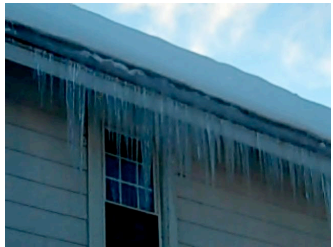
How much bigger until this one causes damage?
