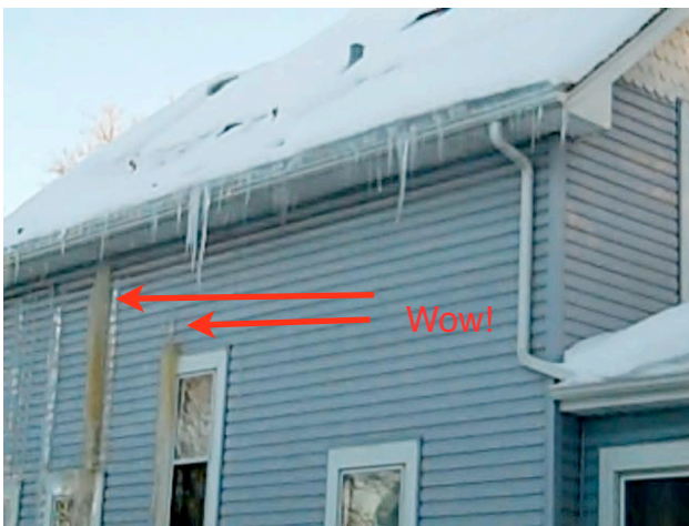
Water/ice flowing out of siding/windows
